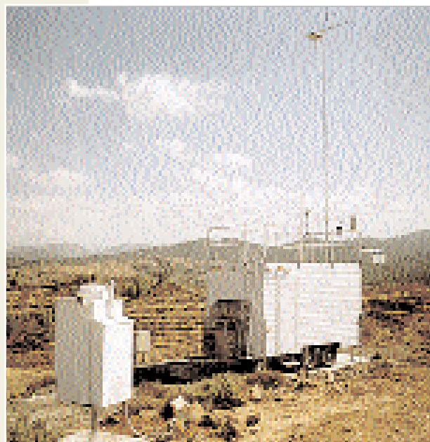
An Ecotech Ambient Air Monitoring installation in Cyprus.
